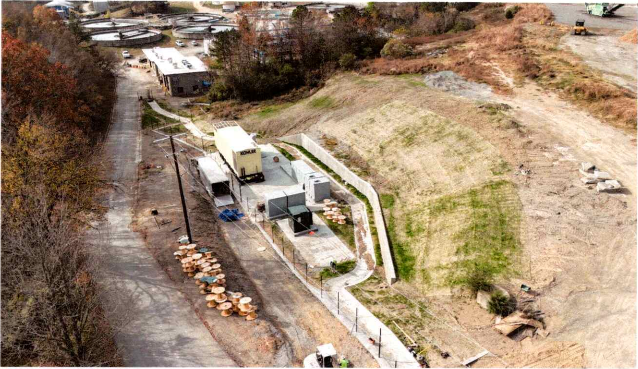
Davidson Drive WWTP Emergency Generator
